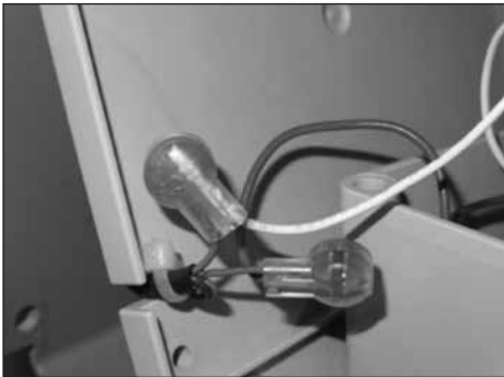
Figure 7.21 - ERT cable properly routed through the back plate
