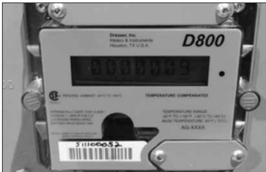
Figure 6.1 - Label on D800 meter
