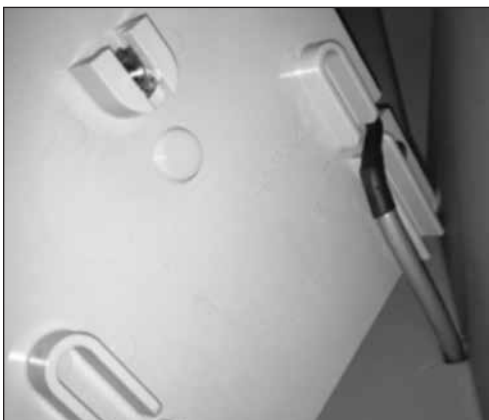
Figure 7.22 - Meter cable routed across back plate
