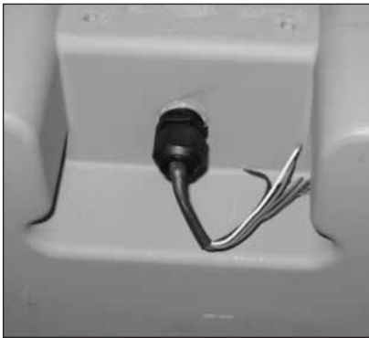
Figure 7.15 - Pulse output cable on backside of meter
