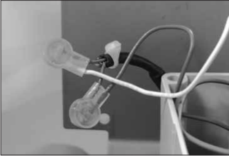
Figure 7.20 - Pulse Output 2 wired to the ERT with a cable tie located near the end of the shrink tubing
